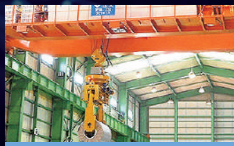
Automatic Overhead Crane
