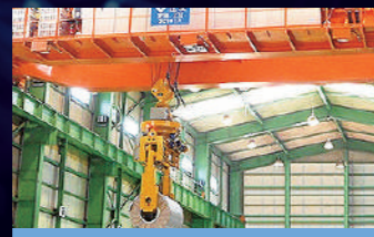
Automatic Overhead Crane
