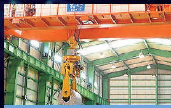
Automatic Overhead Crane
